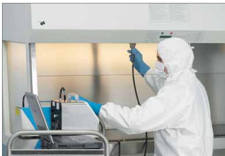
Testing of the HEPA recirculation filter.
